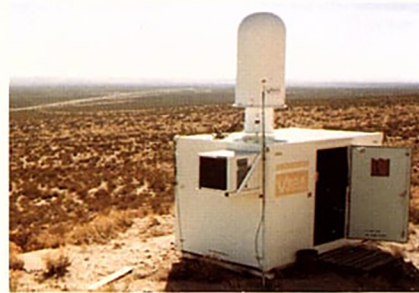
Target Tracking and Control System shelter—range 115 NM (213 km).
